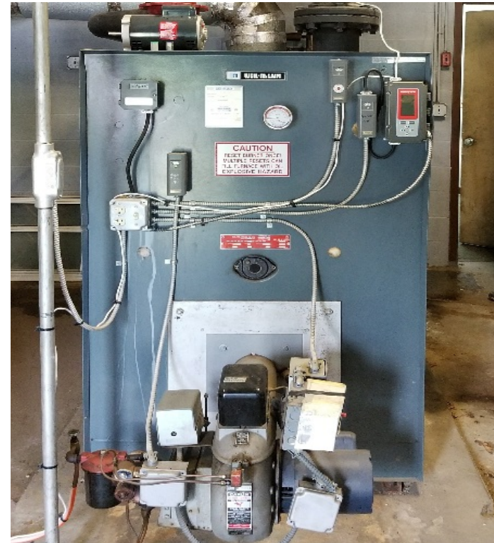
Figure 6.1: The existing boiler at the Smith Government Campus Building 3 will be upgraded with a new gas fuel train and burner.
