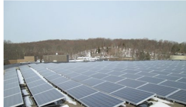
Figure 18.1: Example of a typical ballast mounted solar PV array
